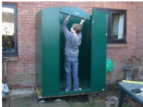
Step 8 The panel over the door is put in place to complete the outside walls.
